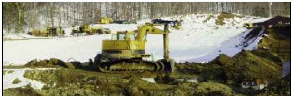
Construction continues on the 27,000 square foot assisted living Alzheimer's residence on the St. John campus.
